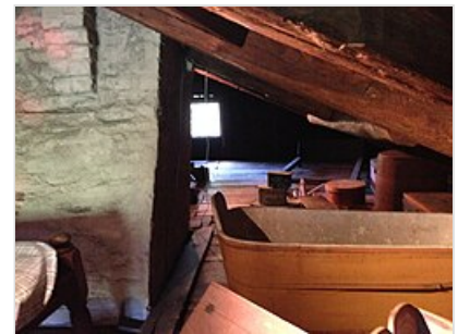
The attic at Fruitlands where Alcott lived and acted out plays at 11 years old. Note that the ceiling area is around 4 feet high
